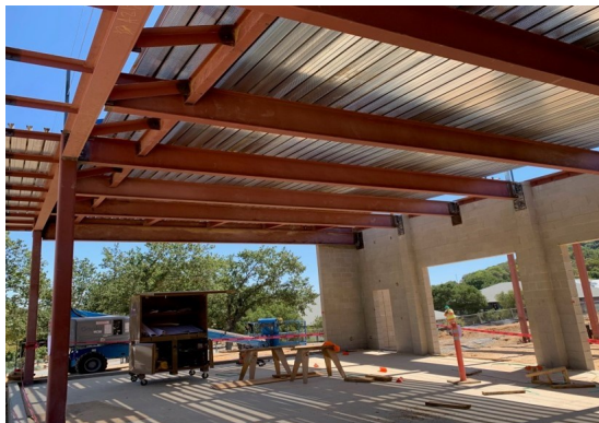
Main Roof Decking and Roofing for New Miwok Center, Indian Valley Campus
